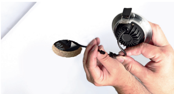
4 - connecting the power supply unit to the spot using a plug connector
